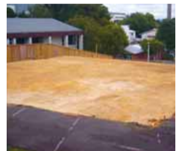
The site for the Tauranga Project Hope centre was cleared in December and blessed, prior to the start of construction.
